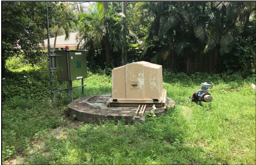
ON-SITE LIFT STATION
